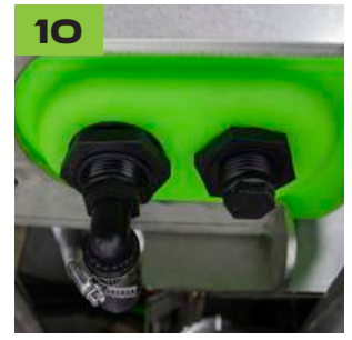
Tank Sump with Drain
